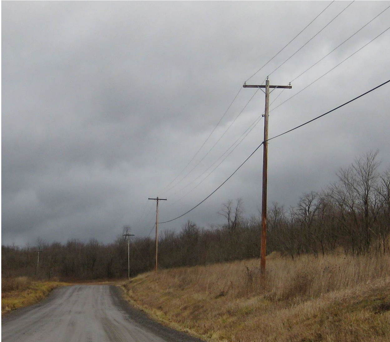
Figure 13: Low-Make-Ready Pole Line in Unserved Area
