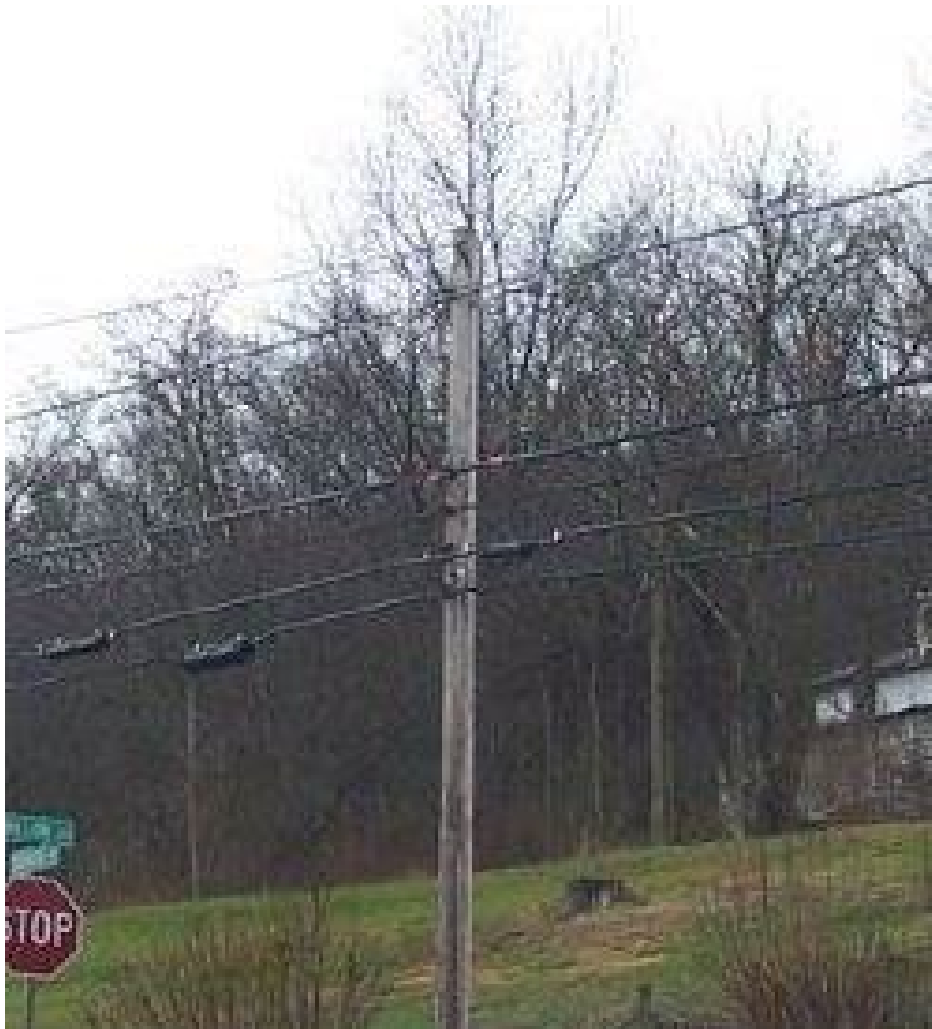
Figure 12: Utility Pole Requiring Make-Ready
