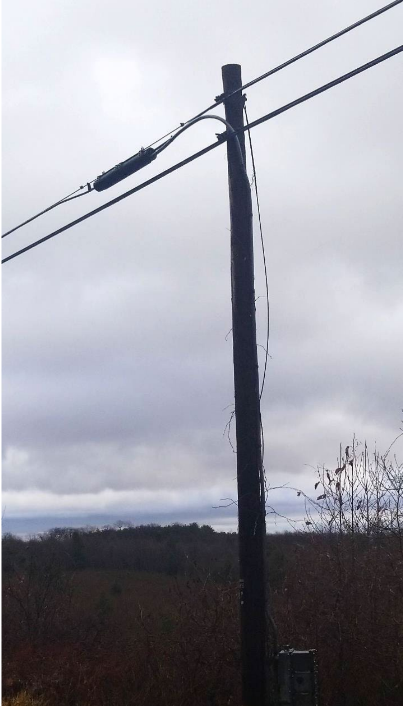
Figure 14: Short Telecommunications Pole
